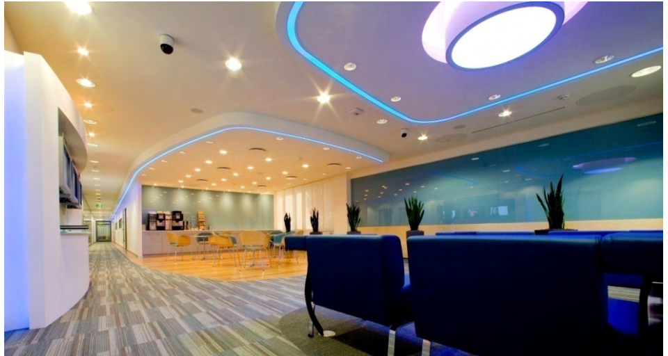
RaumComputer® controls with RC-BOS 400 dimmable Lamps and 160 m LED RGB Lighting
